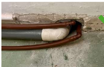
Waste & Overflow Pipes in Floor Drainage Image 13
