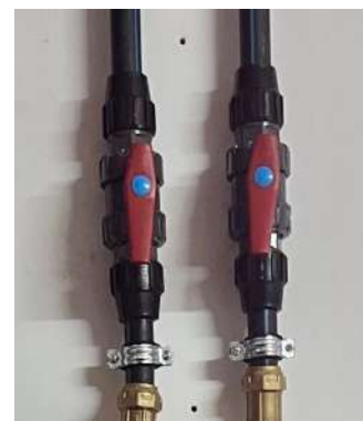
Inlet & Outlet Valves Fully Open Image 23
