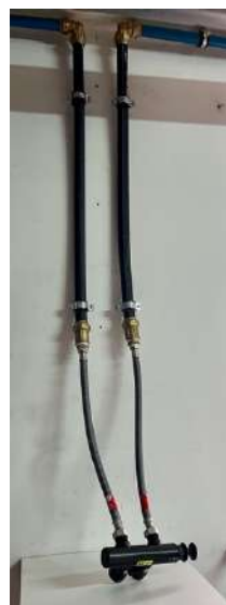
Mains Inlet, Outlet & Bypass Valve Connected Image 17
